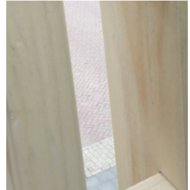
Reddish brown staining
