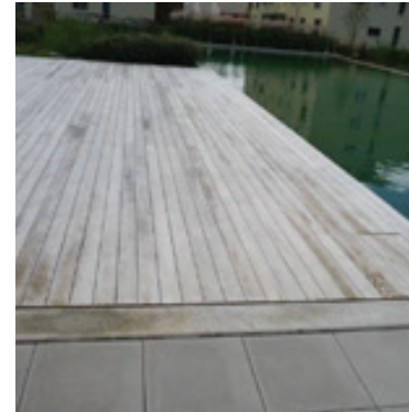
10 months of weathering
